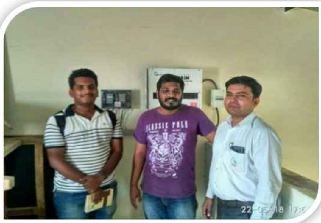
Electric Meter and Net Metering 10 KW project at New Building
