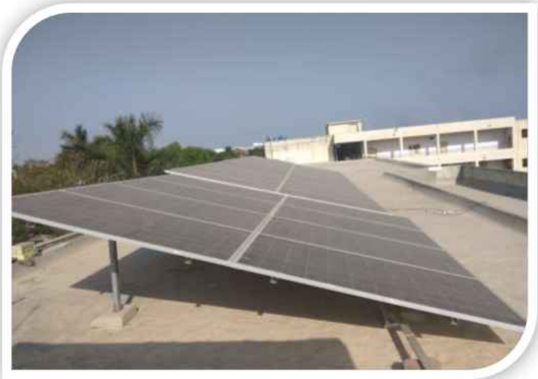
10 KW project under BCUD Savitribai Phule Pune University "Planning and Development Grant
