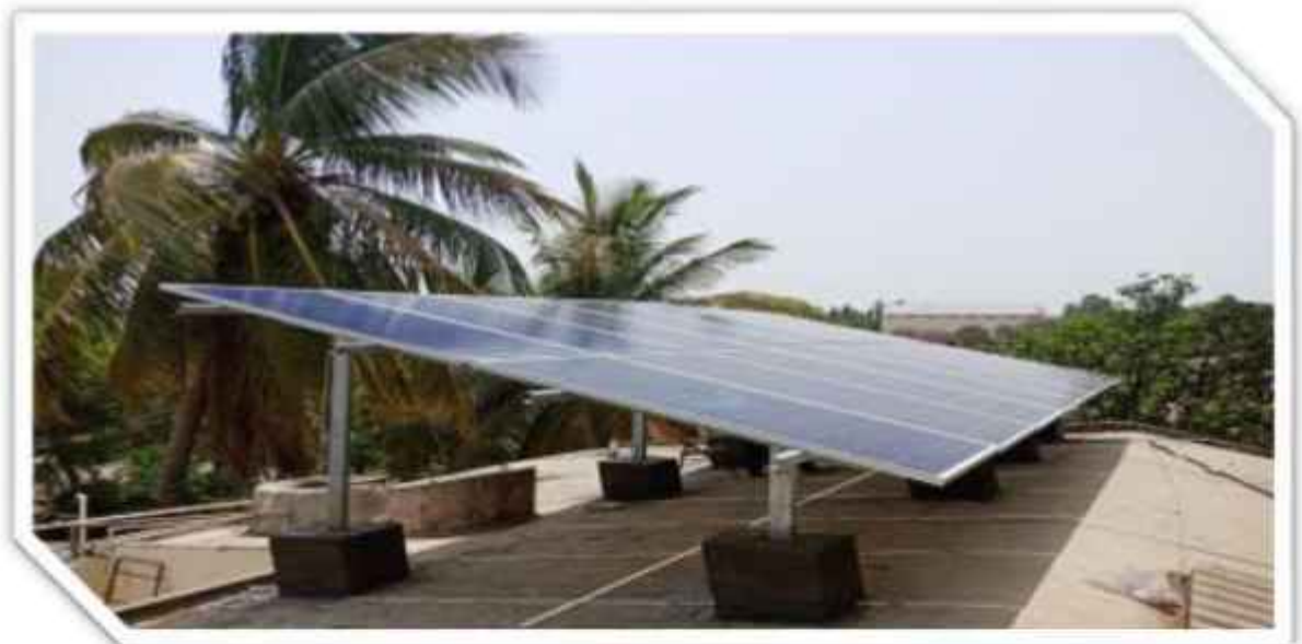
5KW Solar project at Principal bungalow
